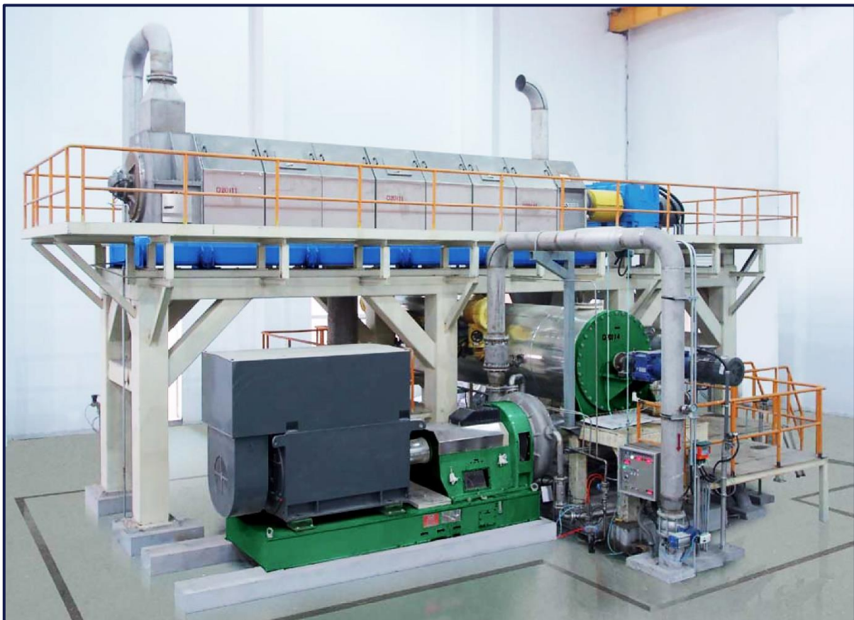
Img. 5. KRIMA system to 500 t/24h
