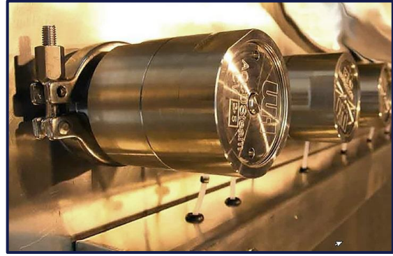
Img.3. Zone control valves
